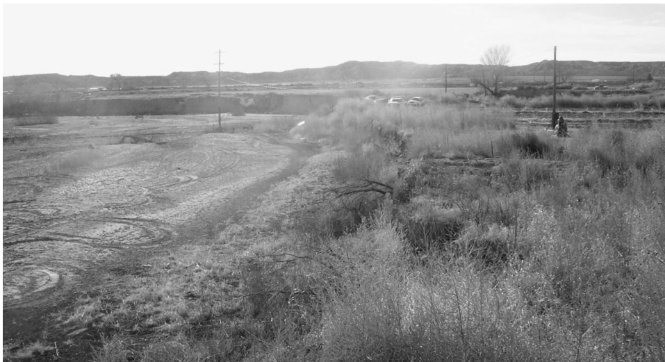
Photograph 2. Eroded South Bank of Gila River where Stateline Road was Washed Out (view southeast). Stacks of concrete-filled tires would be installed in this area to protect the bank from future floods.
